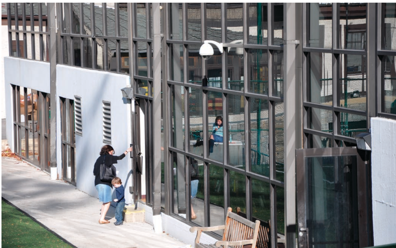
Arecont's 180° megapixel dome camera mounted within view of one of SAR Academy's entrances/exits. The project included the installation of more than 25 new 1.3- to 5-megapixel cameras, which greatly enhance images when compared to the old analog system.
