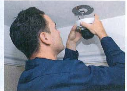
A CSI technician installs one of the hotel's many Sony IP cameras that feed into multiple viewing stations and redundant storage. The system is monitored from a central location on LCD displays as well as other key locations onsite.
