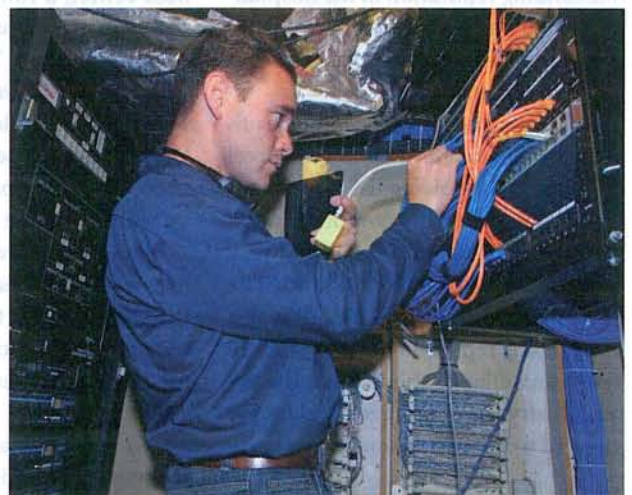
A technician connects the IP system, which CSI designed as a separate, parallel network for security. Cat-6 was used to allow for system growth as well as bandwidth demands exceeding 1GB.
