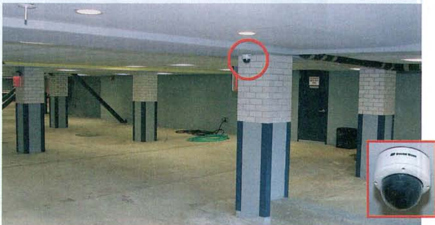
The Allegria's indoor parking garage is equipped with Arecont Vision megapixel cameras to provide the wide field of view desired in that environment.
