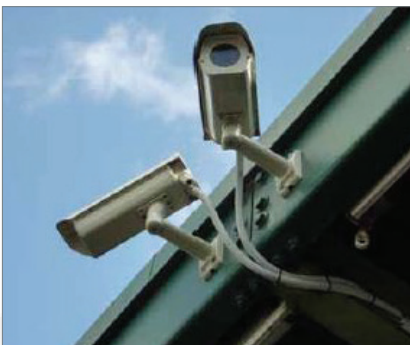
Arecont Vision cameras in weather-resistant housings keep watch on the facility day and night.
