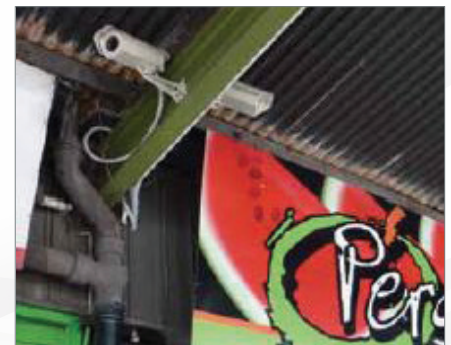
Arecont Vision cameras provide 24-hour surveillance of the large Brisbane Markets loading docks.
