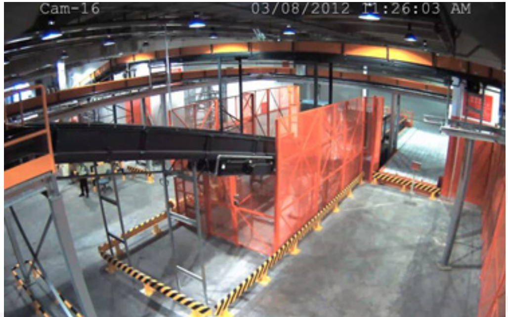
TNT Express chose Arecont Vision megapixel cameras to secure their new 70,000-square-foot facility in Hong Kong.
